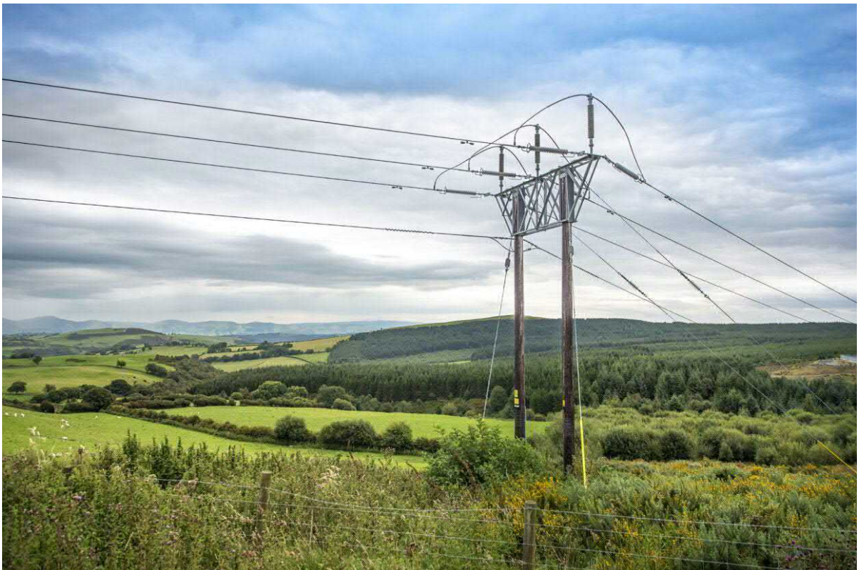
Figure 2.2: Typical back stayed angled 'H' pole where the OHL changes direction
